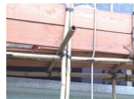
Fig. 1.4 A close-up on the ledger-post connection
