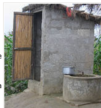
A biogas system attached to an outhouse in Badreni, Nepal. Many villagers are turning to biogas in Nepal, especially as the technology is relatively simple, reliable and accessible. © Trishna Gurung / WWF Nepal
