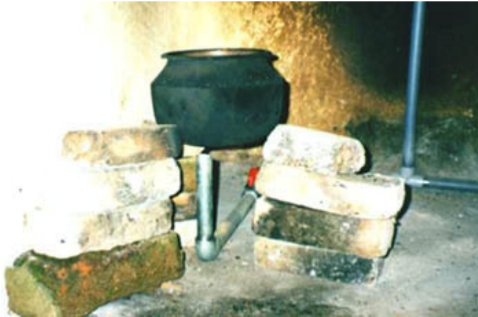
Figure 15. Biogas is brought to the kitchen using PVC connections, due to its corrosive action. Only the last tube is a iron galvanized pipe. A biogas plant can produce enough fuel to fulfill the requirements of a rural family.
