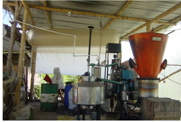
Photo G6: The polyethylene reservoirs suspended close to the gasifier. These are filled with combination of biogas and producer gas. After running the gasifier and engine, the engine is stopped but the gasifier continues to produce gas which is stored in the reservoirs
