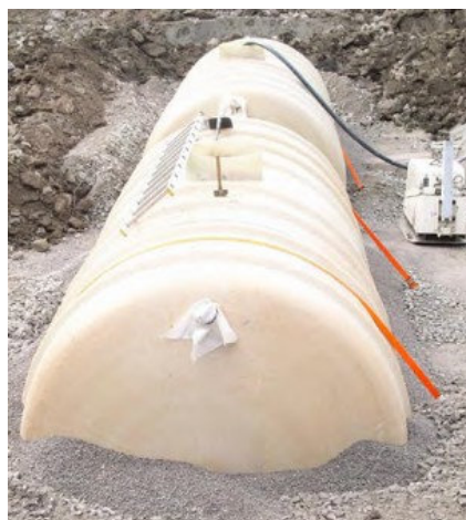
Figure 9. Below-ground plastic urine storage tanks at Kullön, Sweden during the construction process. The tanks will be covered with soil. Photo: Mats Johansson. (Source: Kvarnström et al. (2006), page 36)
