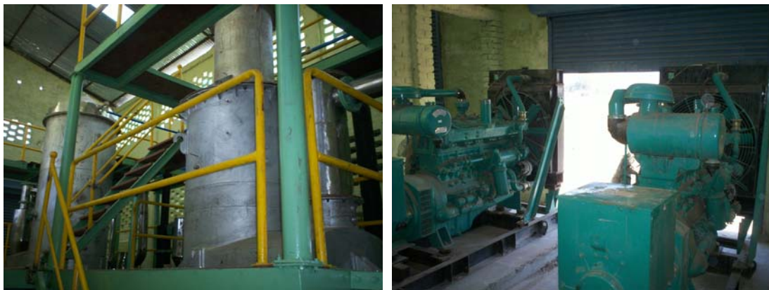
Erected gasifier & gas engine at Gaiyari
